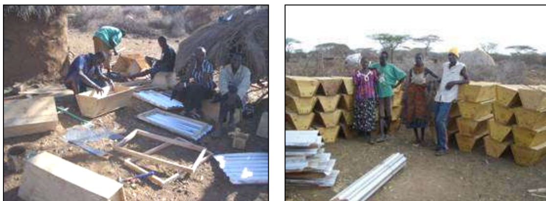
Figure 6.9. (a) The workshop became so busy that activities often spilled outside during the day where several helpers assisted the two carpenters. (b) The beehives were constructed in batches of 50 before being deployed onto the nearby farms.
